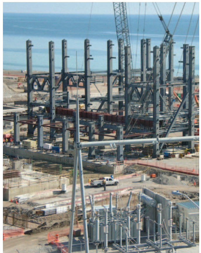
Construction work progresses on two coal-fired power plants in Oak Creek, Wisconsin.
