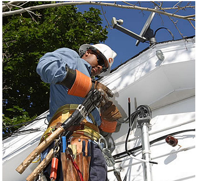
A key component of customer satisfaction is quick restoration of service following storm-related power outages.
