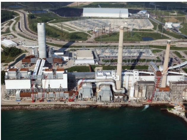
Construction of the Air Quality Control System (AQCS) for the South Oak Creek units.
